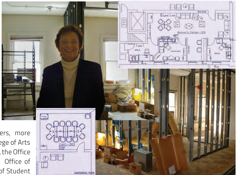
Conversion of Thwing Center third floor space for the new Center offices and a small conference room.
